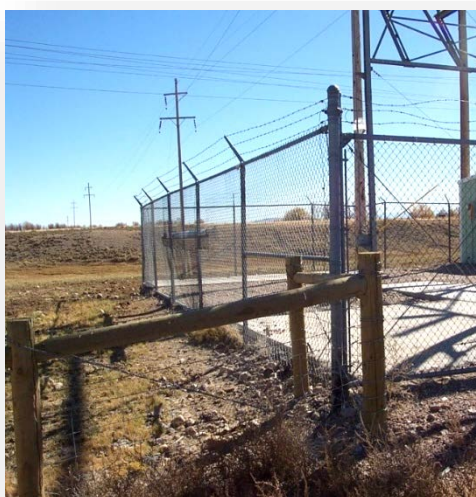
Fencing should never be adjoined to the substation; it can become energized.
