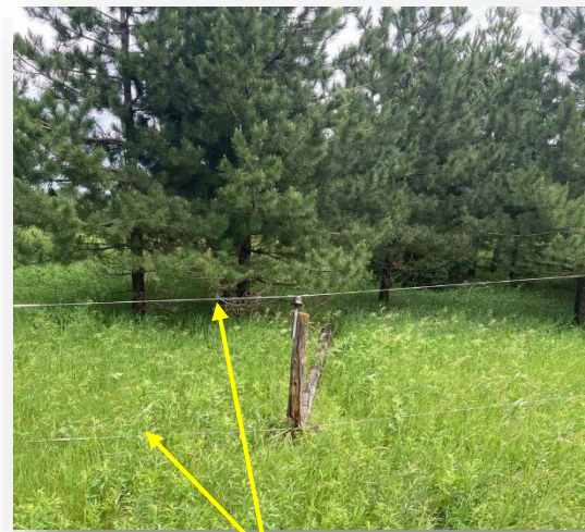
Lines still suspended even with pole broken and on ground (retrieved from Lake Region's Facebook)
